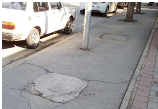
Figure 5. Covered pits of former SUT’s (category 5)
